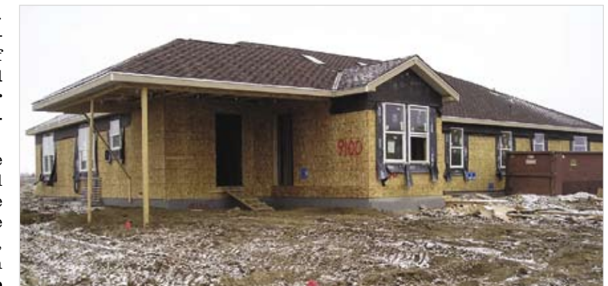
Third Way Center I is well on its way to completion, and will be dedicated this April.
